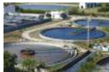
MALAYSIA- SAMALAJU WATER TREATMENT PLANT Merus active filter
