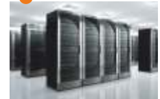
DUBAI- DATACENTER Merus active filter
