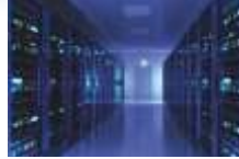
UK- SONY ENTERTAINMENT CENTRE (DATA CENTER) Merus active filter
