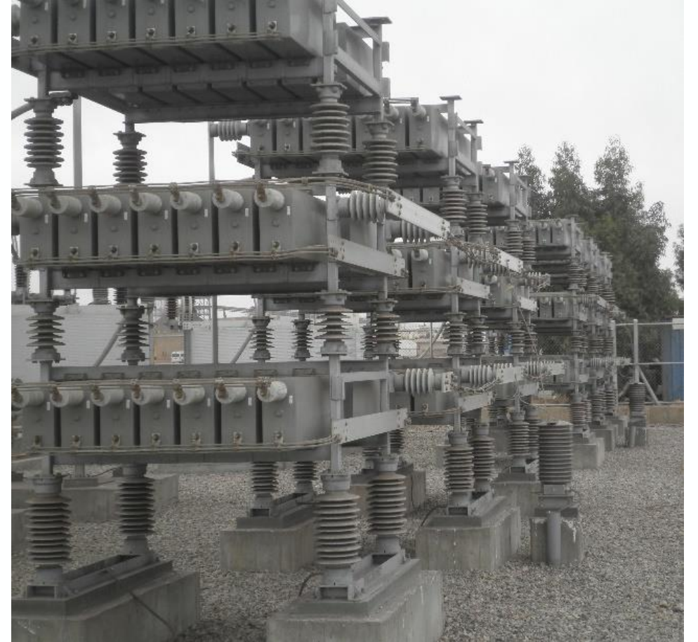
Filter capacitor bank assembly
