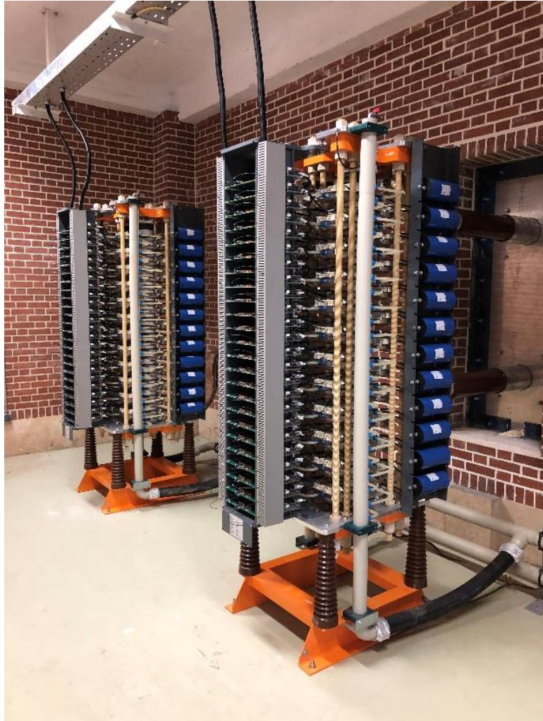
Thyristor valve assembly
