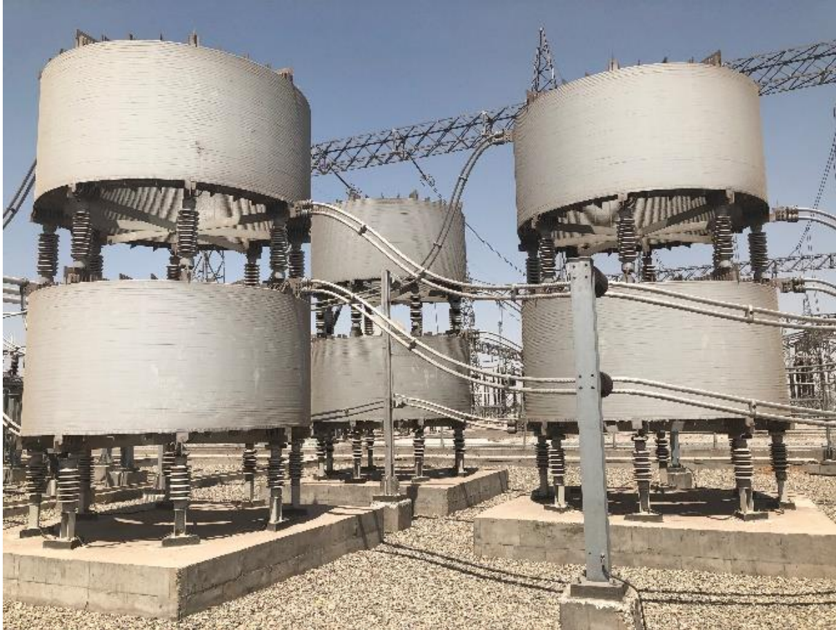
TCR reactor assembly
